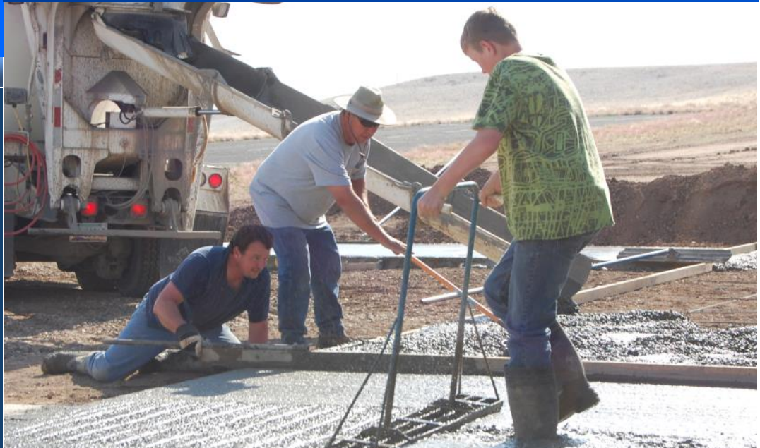
Andy Younker's grandson Ethan is ankle deep in cement as Chris Corbitt, on the ground, and his dad Wes work to level the cement in front of the new field canopy.
