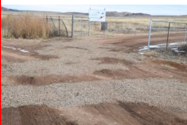
Dale Tomlinson, top photo at right and Steve Shephard smooth out some gravel and fill dirt brought in to fill the nasty pot holes at our gate entry located on the road coming into the flying field.
