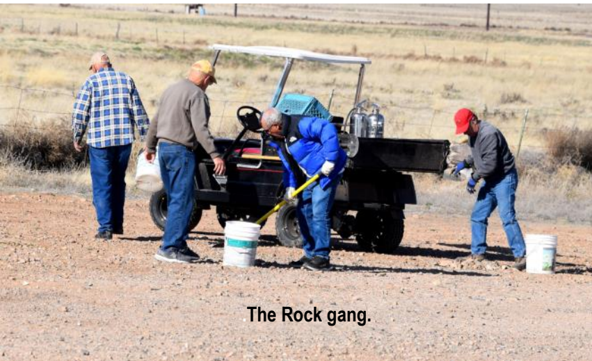
We now have a nice graveled parking area. The drainage ditch that runs in front of the shed has also been cleaned out to improve drainage see photos below.
